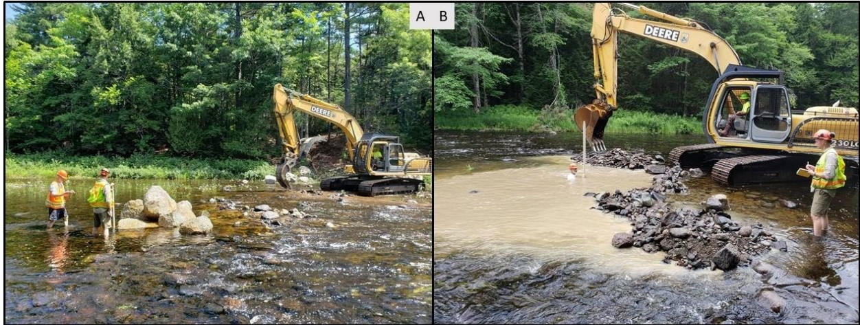
Figure 5.3.8. Restoration work completed at the Route 9 project site, Narraguagus River (2020). Completed boulder clusters and the excavator beginning on the second (A - Left). Engineer measuring the depth an exploratory geotechnical pit (B - Right). (photo credit: Chris Federico, Project SHARE)
