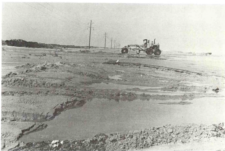
Lower Right Highway damage near Buxton, N.C. Photo courtesy Ray Couch and Dare County Tourist Bureau.
