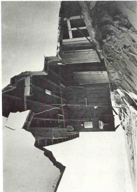
Wind-driven waters washed away the sand from under this Kitty Hawk, N.C. cottage.
