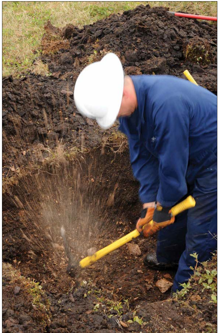
Coast Guard Chief Petty Officer James Brumley prepares a site for the installation of an Aids to Navigation tower south of Point Hope, Alaska, in 2010. For a blue economy to succeed, a robust communications infrastructure, among other infrastructure improvements, is crucial. Coast Guard photo by Petty Officer 3rd Class Walter Shinn
