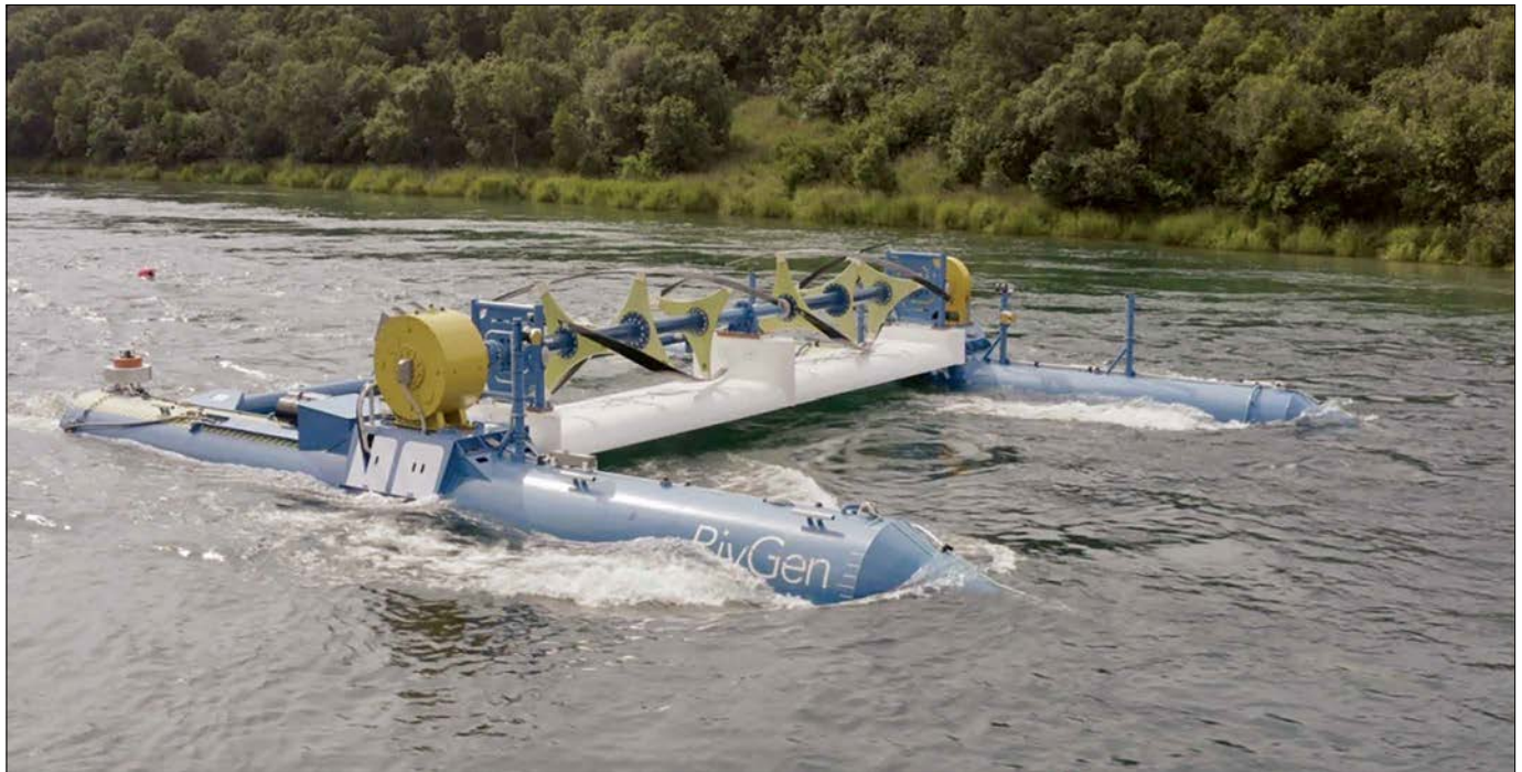
In June 2019, the RivGen Power System was installed on the Kvichak River in Igiugig, Alaska. Developed by the Ocean Renewable Power Corporation, the turbine is engaged by the river's water current and distributes electrical power via a cable connected to the village's power grid. Photo courtesy of the Ocean Renewable Power Corporation
