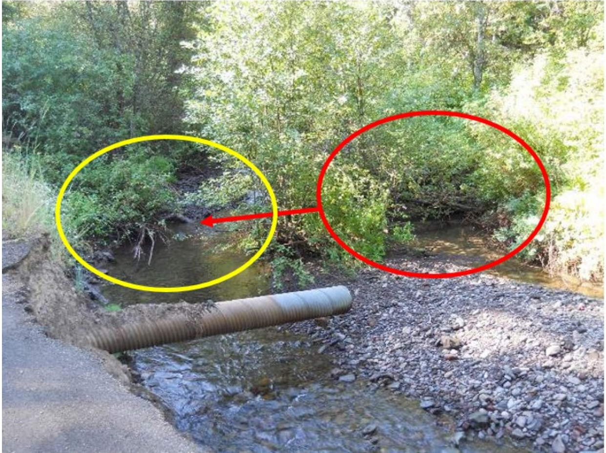
Figure 2. Picture of LWD accumulation that WWNF will relocate from river left (red circle, existing location) to river right, proposed location). WWNF may choose to excavate the secondary channel downstream of the red circle to recreate the main channel.
