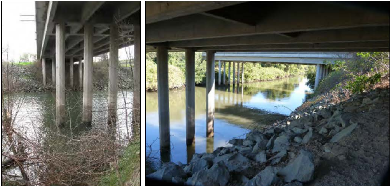
Figure 1. Mokelumne River Bridges eastern and western spans. Bents shown are bents 4 and 5 which are near or below the ordinary high water mark (from Caltrans 2016).
