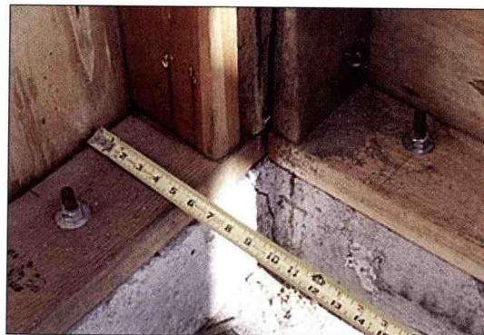
Figure 2. Properly bolted bottom plate. However, note the weak straight-nailed connection between the wall studs and bottom plates.
