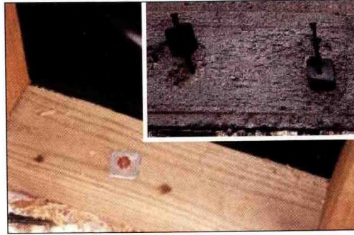
Figure 7. Shot pin with attached washer in the bottom plate. Inset photo shows aftermath of tornado where bottom plate broke around the fasteners.
