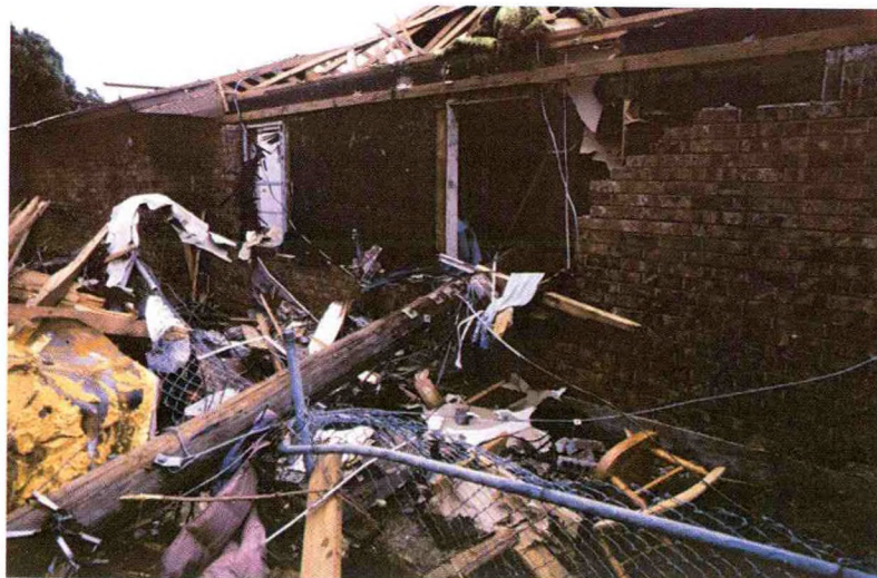
Figure 30. A power pole propelled through a window during the 3 May 1999 tornado in Del City, Oklahoma. It clearly did not tip over and through the window, since the top of the window frame remains intact (FEMA photograph by C. Doswell).
