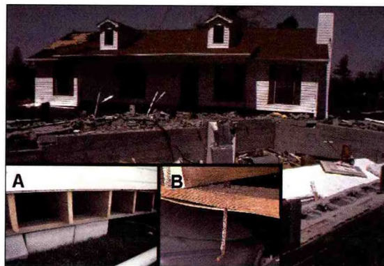
Figure 15. This home shifted off its foundation when the masonry foundation failed. Inset photograph A shows that the top row of masonry was attached with J-bolts as shown in inset photograph B. Note how little damage there was to the roof.
