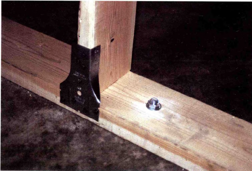
Figure A2.6. Example of a metal clip reinforcing the attachment of wall studs to the bottom plate. Note the bottom plate is bolted to the foundation with a nut and washer. [Photograph © T. Marshall, used by permission]
