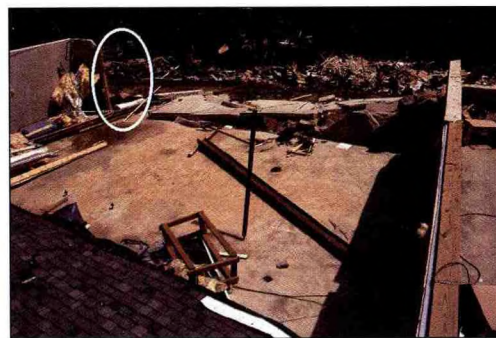
Figure 13. Exit door weakened the concrete wall foundation (circled). The foundation wall rotated and broke apart at the opposite corner. Steel rebar was used only at the wall corners. The house was pushed into the ravine in the background.
