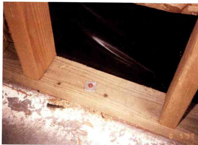
Figure A2.2. Attachment of bottom plate by shotpins. [Photograph © T. Marshall, used by permission]
