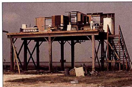
Figure 18. Wind damage to a home elevated on timber piles. Failure commonly occurs where the walls are attached to the floor.
