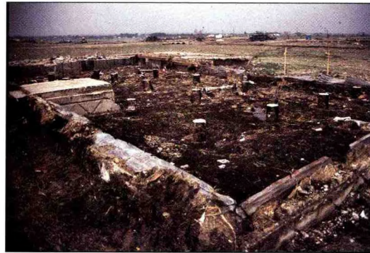
Figure 10. This home shifted and disintegrated from its wooden pier and concrete beam foundation. Floor joists were not attached to the piers.
