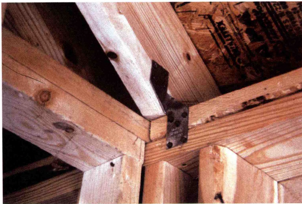
Figure A2.8. Example of a metal clip reinforcing the attachment of the roof trusses to the top plates. [Photograph © T. Marshall, used by permission]
