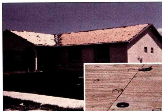
Figure 26. Poor installation of the roof covering on this home led to its complete removal. Staples were installed crooked and under-driven (inset photograph).
