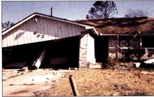
Figure 21. Inward failure of garage door led to outward failure of sidewall and collapse of the garage. Note little damage to remainder of home.
