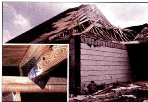
Figure 24. Topped roof trusses due to a lack of lateral bracing. A metal bracket (inset photograph) along with proper wooden blocking between the trusses would have prevented rotation of the trusses.
