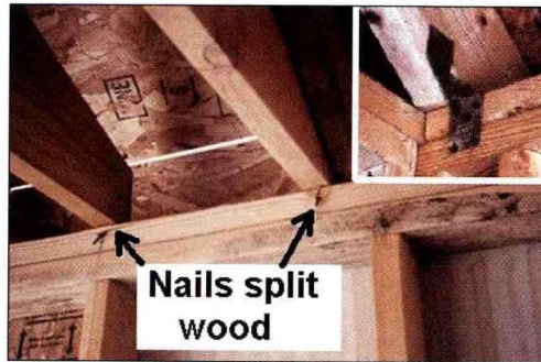
Figure 23. Nails driven through rafters and ceiling joists protruded through the top plate and split the wood. A better connection would have been to install metal clips as shown in the inset photograph that places the nails in shear (strong) instead of tension (weak).
