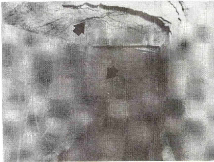
Photo 5. Collection gallery at 90° turn shows steel baffle plate and rough concrete ceiling at Little Goose Dam.
