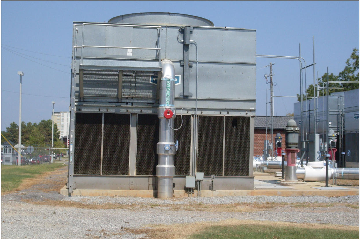
Figure 3-E. View of chiller units, looking north from northeast corner of site. Date taken: 9/21/2010
