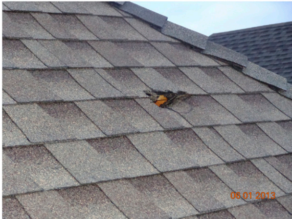
FIG. 2. Photograph of a hole in the roof of a house impacted by a 13-cm hailstone (photo taken by D. Meyer; used with permission).
