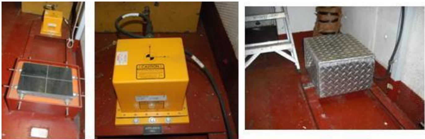
Figure 2. Photos: Clockwise from left: IMU and granite block, IMU, IMU under protective housing. All photos in fan room.
