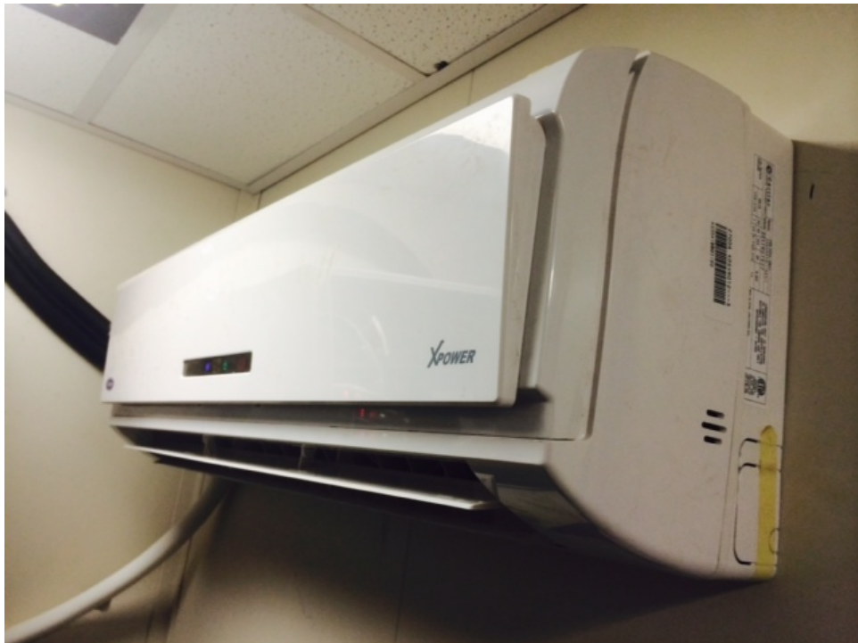
Figure 5. Sonar closet AC unit installed 2015. 2 of 2 units.
