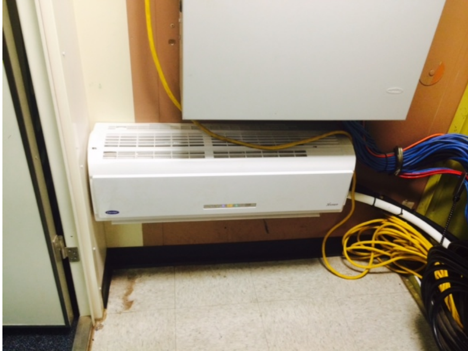
Figure 4. Sonar closet AC unit installed 2015. 1 of 2 units.
