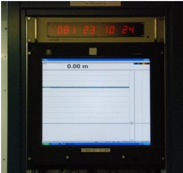
Figure 5. Photo of EA 600 RDS controller in the Dry Lab computer rack.
