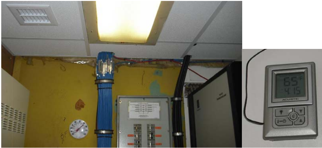
Figure 5. Temperature gauges installed 2009/2010 winter inport.
