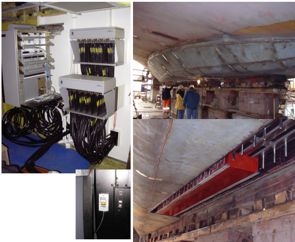
Figure 4. (Clockwise from left) EM 302 TRU unit, Transducer fairing, Elements of EM 302 being installed inside the fairing, TRU remote on / off switch.
