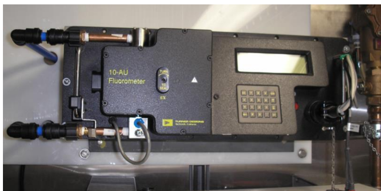
Figure 8: Turner designs 10-AU installed in wetlab.
