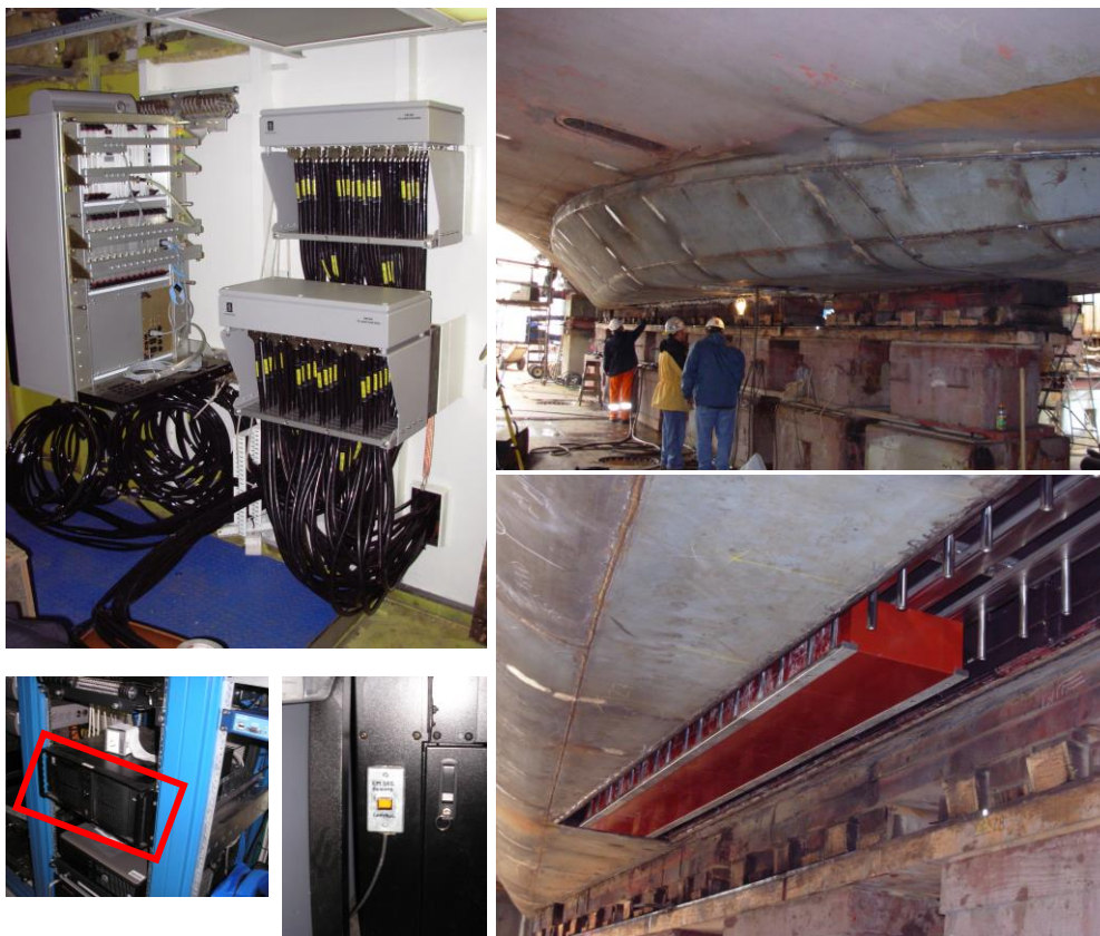
Figure 3: (Clockwise from left) EM 302 TRU unit, Transducer fairing, Elements of EM 302 being installed inside the fairing, TRU remote on / off switch, EM 302 EM 302 SIS control computer.
