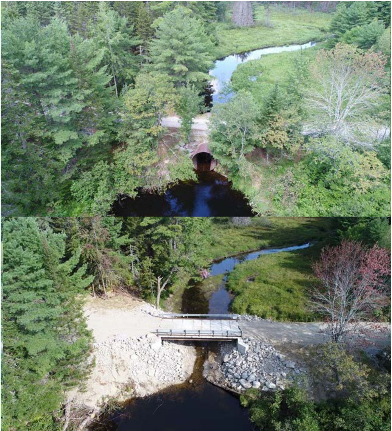
Figure 5.3.2 West Branch Brook culvert replacement, before (top) and after (bottom), Narraguagus River, Maine, 2018. (photo credit: Chris Federico, Project SHARE)
