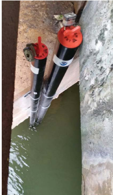
Figure 5. Photograph of turbidity logger (right) and level logger (left) housings attached to the Ajayan River bridge abutment.
