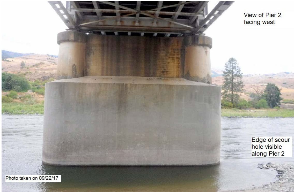
Figure 3. View of Doumecq Bridge Pier 2 with visible scour hole (COE 2019).
