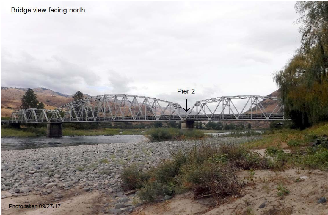
Figure 1. View of Doumecq Road Bridge facing north. Photo taken during Idaho Transportation Department's bridge inspection on September 27, 2017 (COE 2019).
