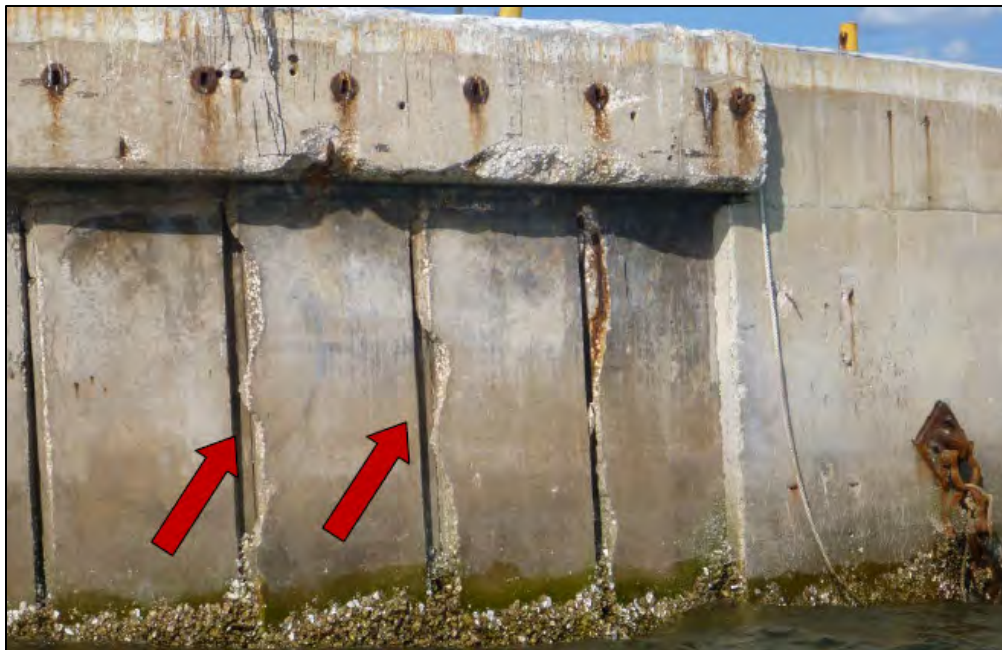
FIGURE A-2. VIEW OF THE TYPICAL SECTION LOSS ALONG THE EDGES OF THE PRECAST CONCRETE PANELS OF THE WHARF CAP NEAR STATION 0+90, LOOKING NORTHEAST
