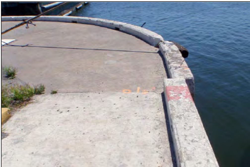
FIGURE A-4. VIEW OF SOUTHEASTERN CORNER OF DECK – NOTE DISLOCATION OF THE BULL RAIL
