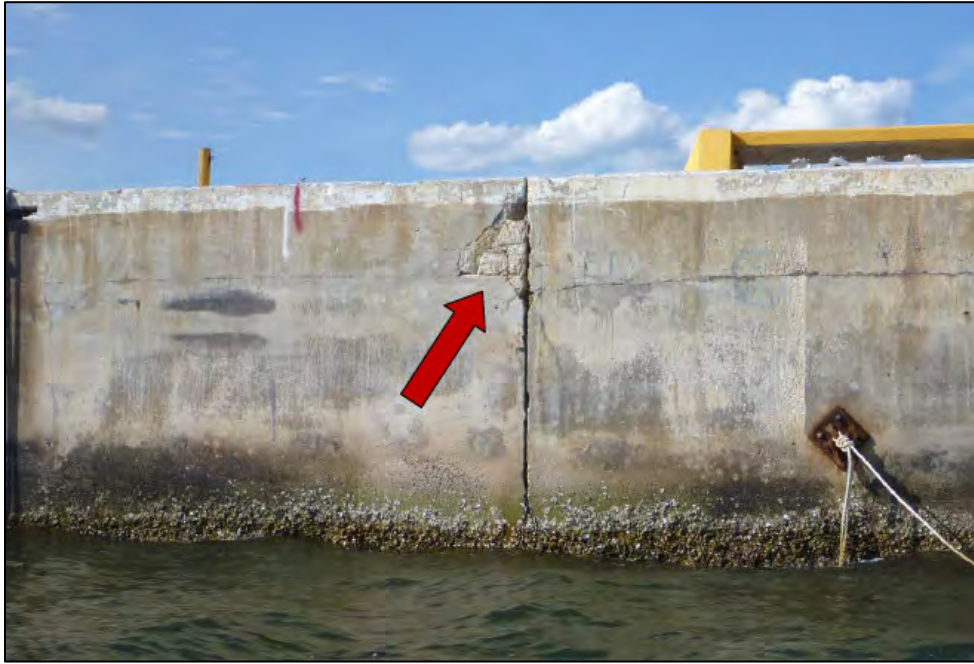
FIGURE A-1. VIEW OF A MINOR AREA OF CONCRETE DETERIORATION IN THE CONCRETE CAP ALONG THE CONSTRUCTION JOINT NEAR STATION 5+50, LOOKING NORTH
