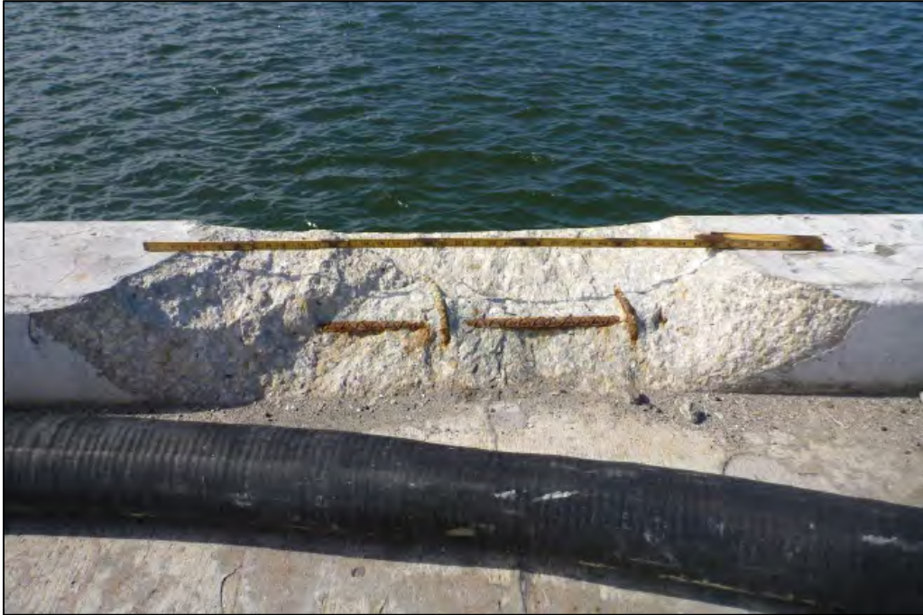
FIGURE A-3. VIEW OF THE SPALL ALONG THE CONCRETE CURB AT STATION 4+40 THAT WAS 3 FT LONG BY 12 IN. WIDE BY 8 IN. HIGH WITH EXPOSED AND CORRODED REINFORCING STEEL, LOOKING SOUTH
