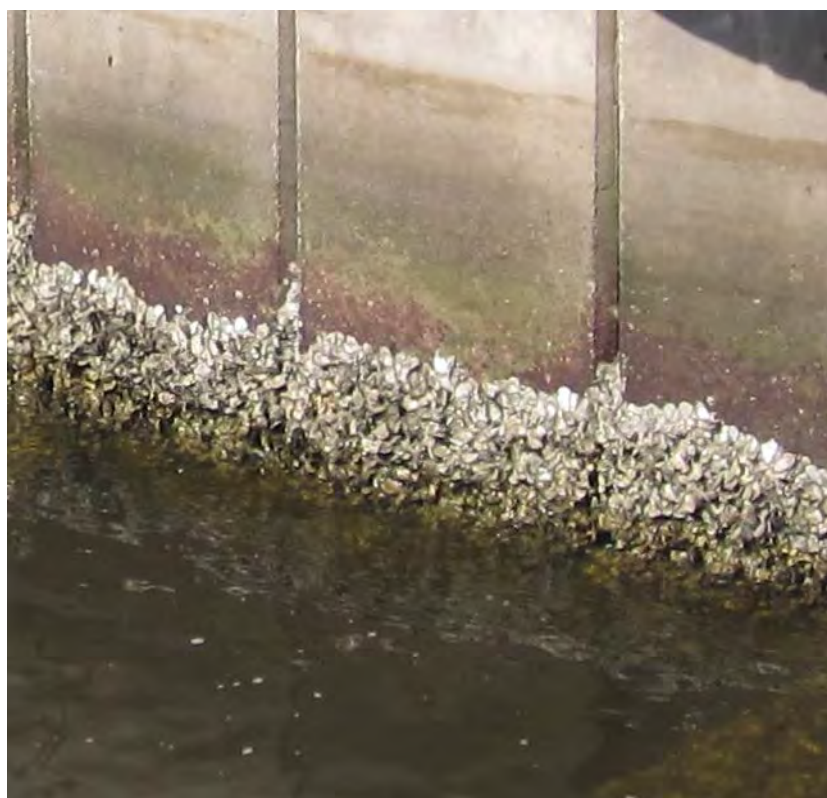
Figure 3-5. Vertical oyster reefs visible on photograph of the Wharf C-2 curtain
