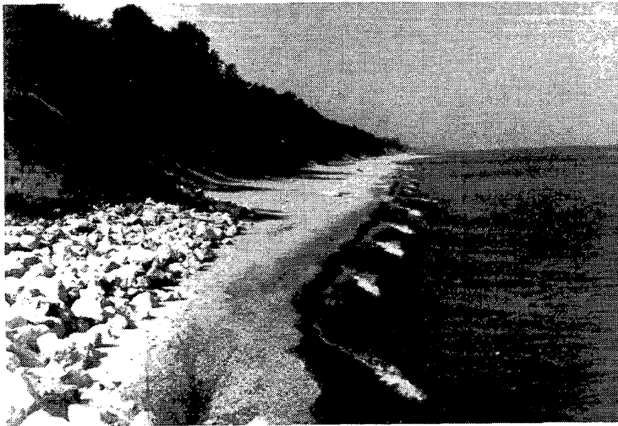
Figure B2. Site A: Looking along beach in a southerly direction from revetment just north of property. What appears to be groin ends is actually the end of the second tier of bags and groins extend into the water.
