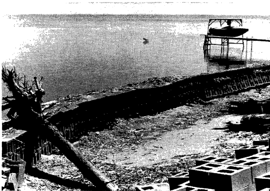
Figure B66. Site Z: Backside of sandgrabber wall, sand level behind slightly higher than in front. Also note tree trunk washed over wall during high water.
