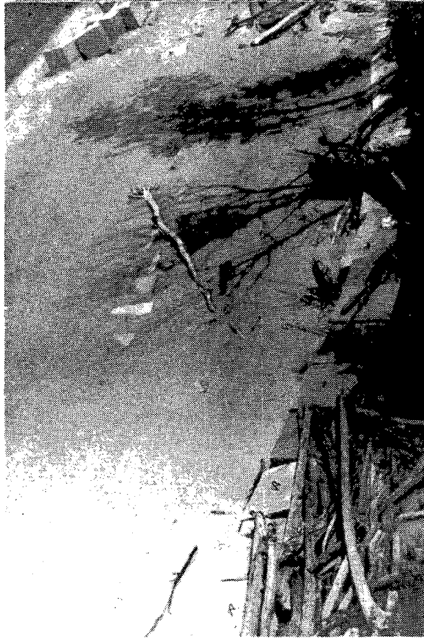
Figure B5. Site B: View of concrete blocks towards southern side of property. Note row of blocks at right, located at toe of bluff. A second row is almost completely buried in the sand to the left of the first row and a few random blocks such as those in upper left have been recently placed on existing beach.
