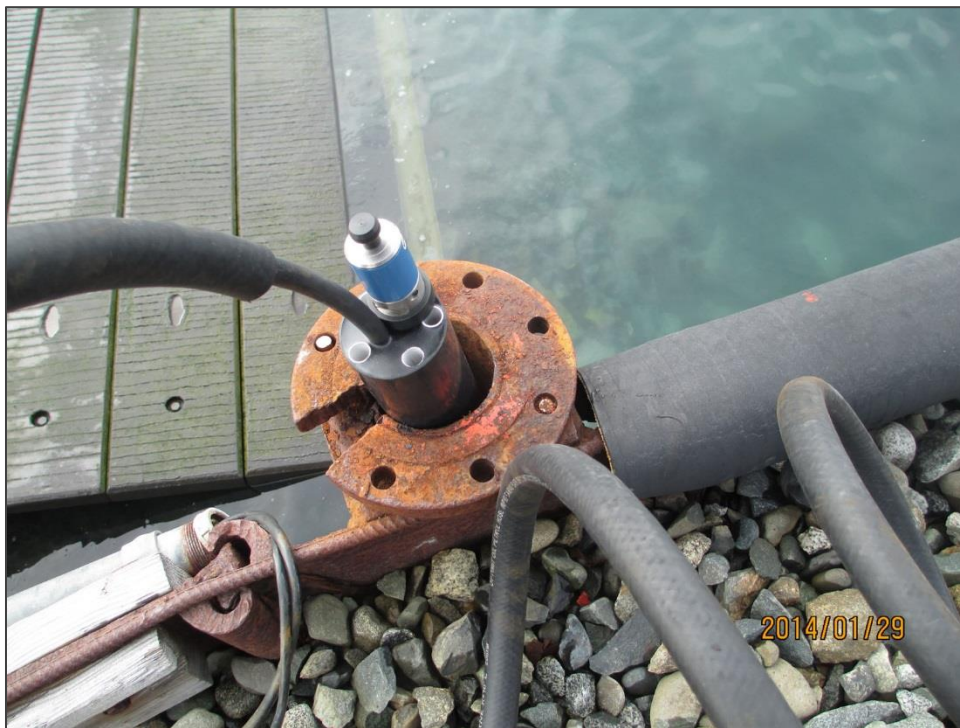
Figure 2-5. An Aanderaa 5218 pressure sensor is lowered into a protective well, providing single point, non-directional wave observations. (Photo courtesy of Richard Butler/Aanderaa)
