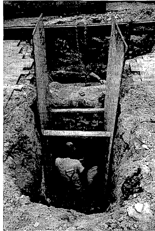
Figure 3-8(a). Excavation of the reentry manhole location. The concrete Virginia Power duct can be seen in the center. The Bell Atlantic duct is behind the Virginia Power duct and cannot be seen from this angle.
