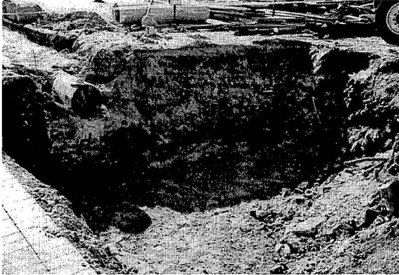
Figure 3-6(b). Excavated site of the filter structure. There are brick foundations exposed along this wall. The pipe to the left runs from the diversion manhole to the Carbon/Sand Filter.
