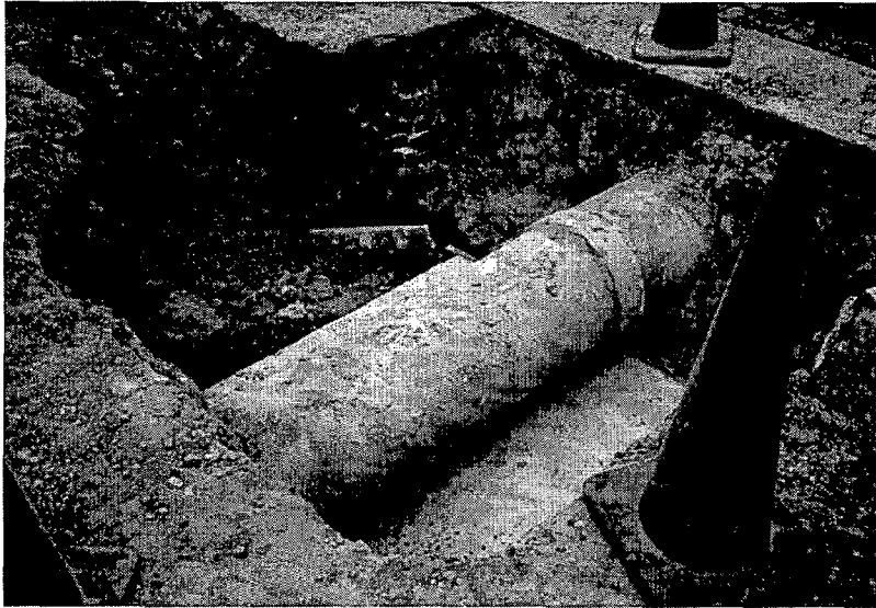
Figure 3-7(a). Construction of the diversion manhole. The footing was poured under the original storm drain pipe carrying drainage from the asphalt parking lot. Note the exposed brick foundations.
