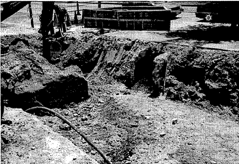
Figure 3-6(a). Excavation of the filter structure location. Note the exposed brick foundation on the left and the concrete foundation just right of center. The wooden barriers in the background protect the reentry manhole.
