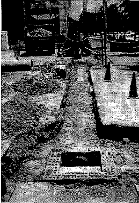
Figure 3-7(c). The view from the diversion manhole toward the Carbon/Sand Filter, not yet constructed.
