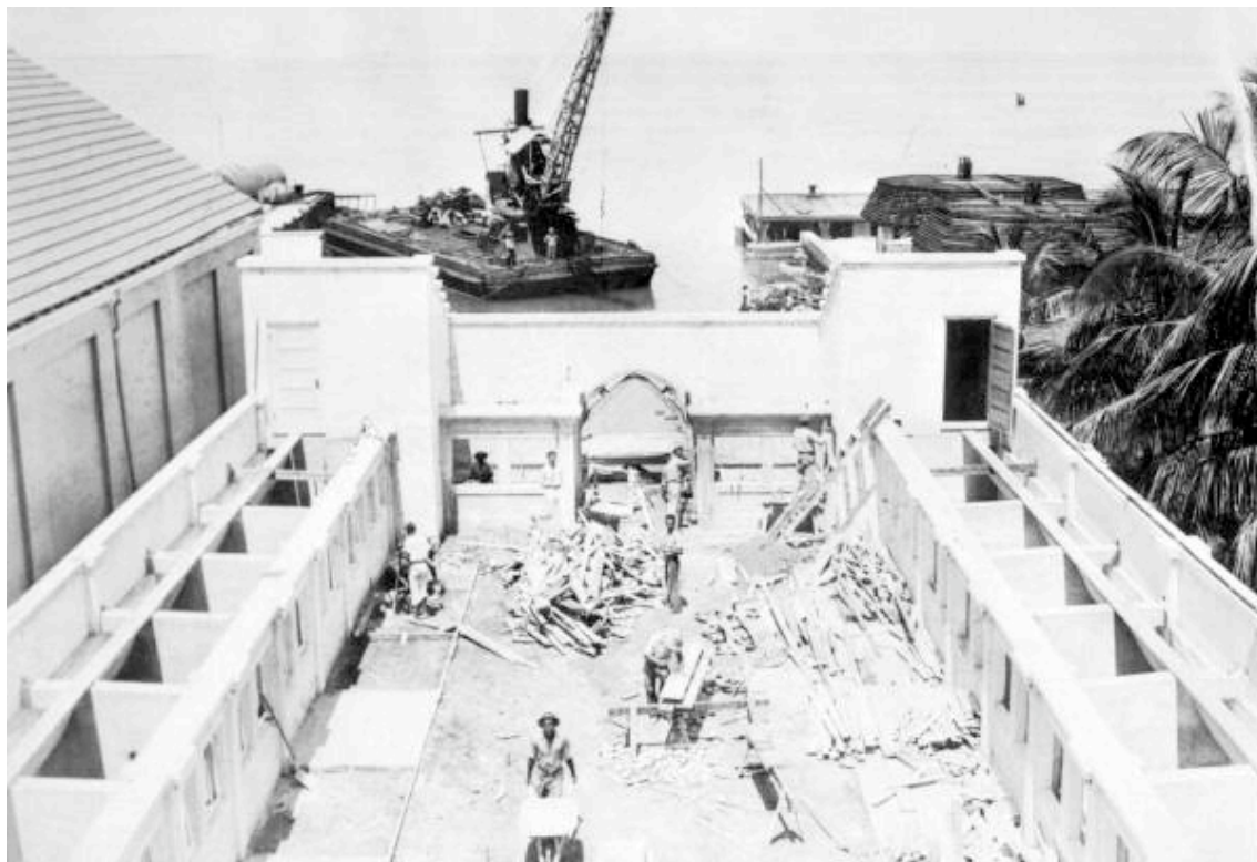
Plate 5. Construction of an open-air aquarium (1935) [Photonegative, black and white (3 x 5 in). PR06058. Print Collections, Florida State Photo Archive. < http://fpc.dos.state.fl.us/ >.]
