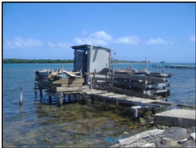
Toilets and pig pens release sewage directly into the lagoon
