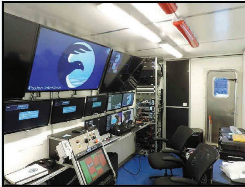
ROV Control Van Interior
