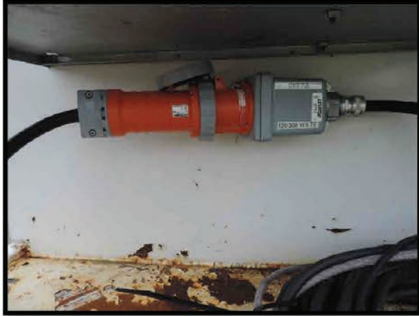
Workshop Van power connection (located at Control Van)
