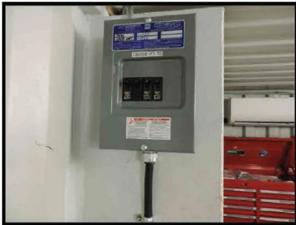
Workshop Van power distribution panel
