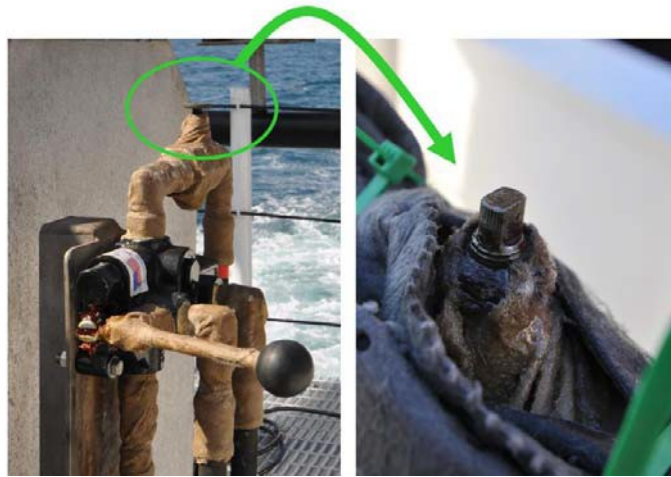
Figure 3. Photo of Winch Speed Adjuster (prior to failure) and close up of poor screw condition and leak.
