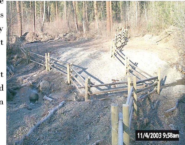
A hardened access point gives livestock a way to reach a short segment of a stream where they can water without damaging the system as a whole. (Photo courtesy of Natural Resource Conservation Service)
