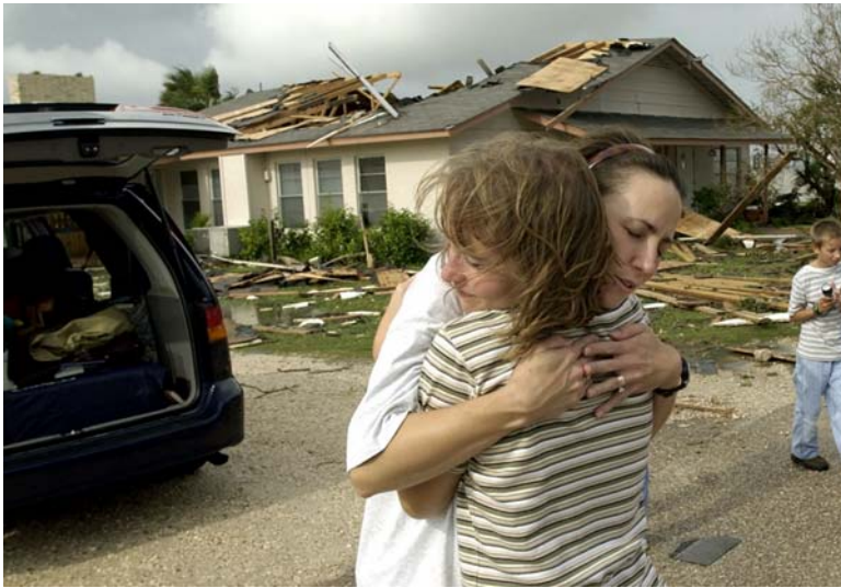
Hurricane Claudette came ashore in Texas on July 15, 2003, peeling off roofs of homes such as this one in Palacios, Texas, knocking out power and flooding low lying areas. (AP Wide World Photos)
