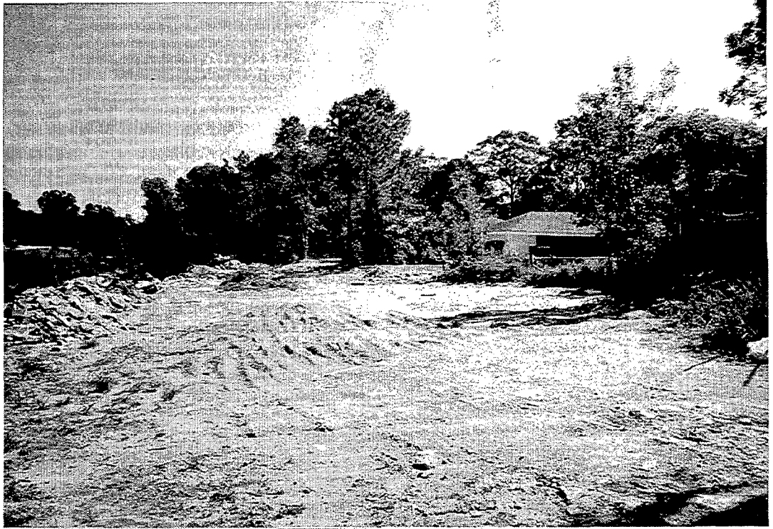
NORTH BRANCH WARD CREEK-BANK FAILURE AND ATTEMPTED RIP-RAP AND FILL REPAIR
