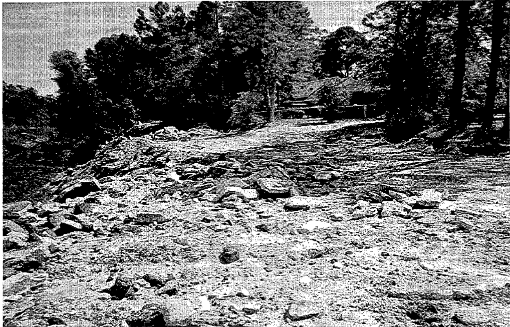
NORTH BRANCH WARD CREEK-BANK FAILURE AND ATTEMPTED RIP-RAP AND FILL REPAIR
