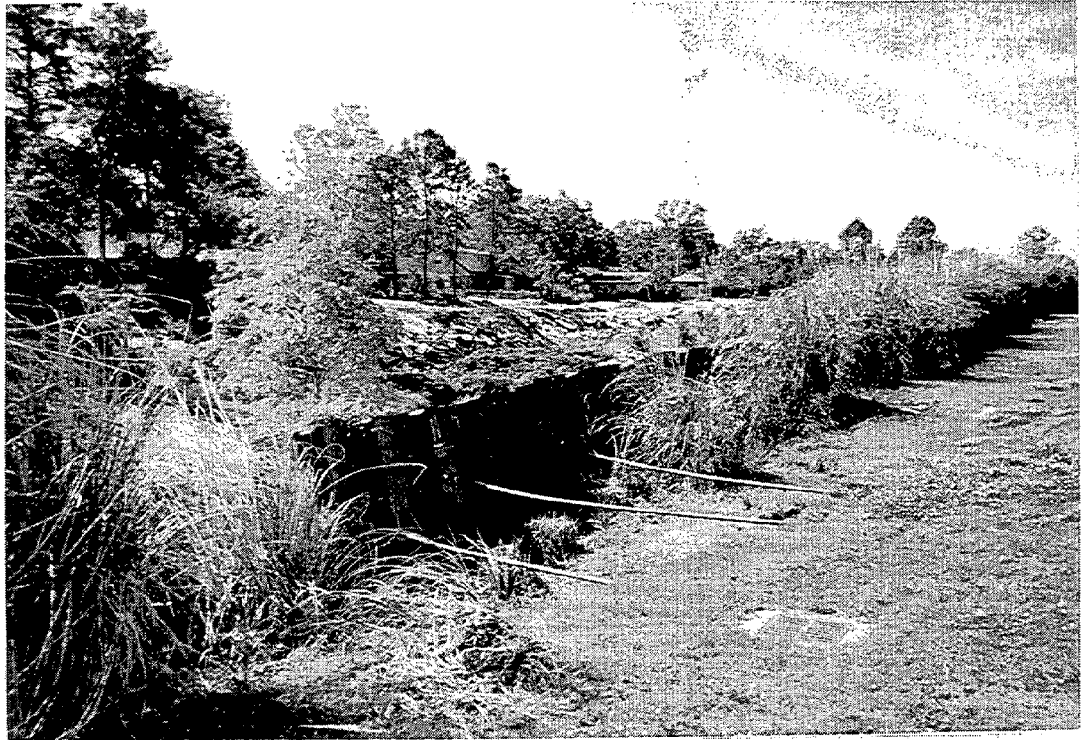
NORTH BRANCH WARD CREEK-SHEETPILE RETAINING WALL FAILURE
