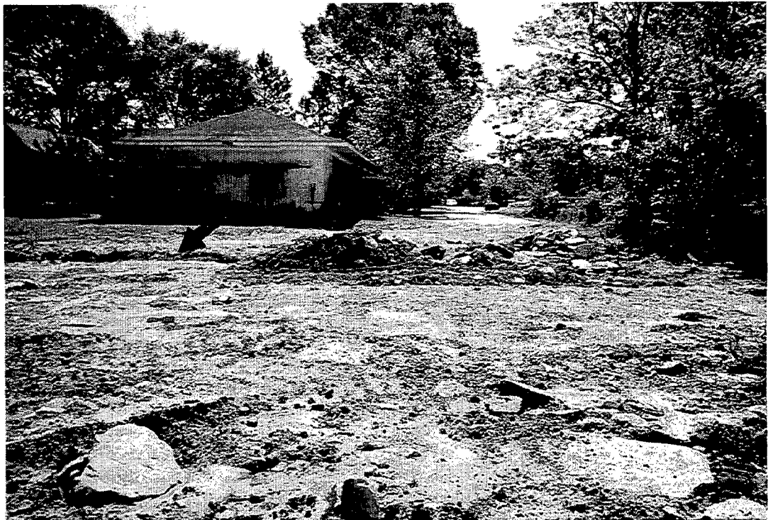
NORTH BRANCH WARD CREEK-BANK FAILURE AND ATTEMPTED RIP- RAP AND FILL REPAIR; NOTE NEW FAULT CLOSER TO STRUCTURE
