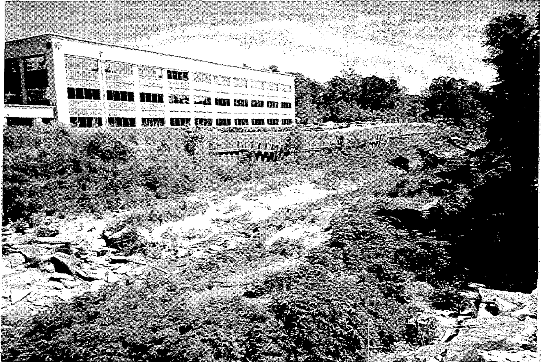
NORTH BRANCH WARD CREEK-BANK FAILURE AND ATTEMPTED SHEETPILE REPAIR
