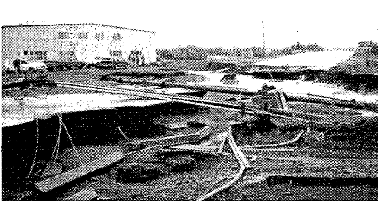
Figure 2b. Erosion damage in Seward that cut through a street and exposed utility lines.
