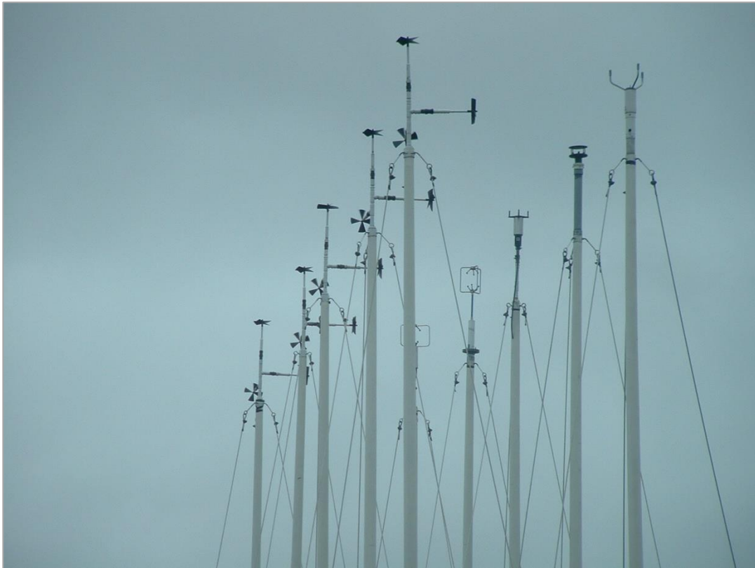
Figure 2-4. Acoustic anemometers at the Otis Weather Test facility in Cape Cod, Massachusetts. The five masts on the left provide reference wind observations. The five sensors on the right are: 1) RM Young 3-axis ultrasonic anemometer (partially obscured), 2) Gill R3 3-D anemometer, 3) RM Young 2-axis ultrasonic anemometer, 4) Gill Windsonic 2-axis ultrasonic anemometer, and 5) Vaisala WS425 ultrasonic anemometer (photo courtesy of Mark Bushnell).
