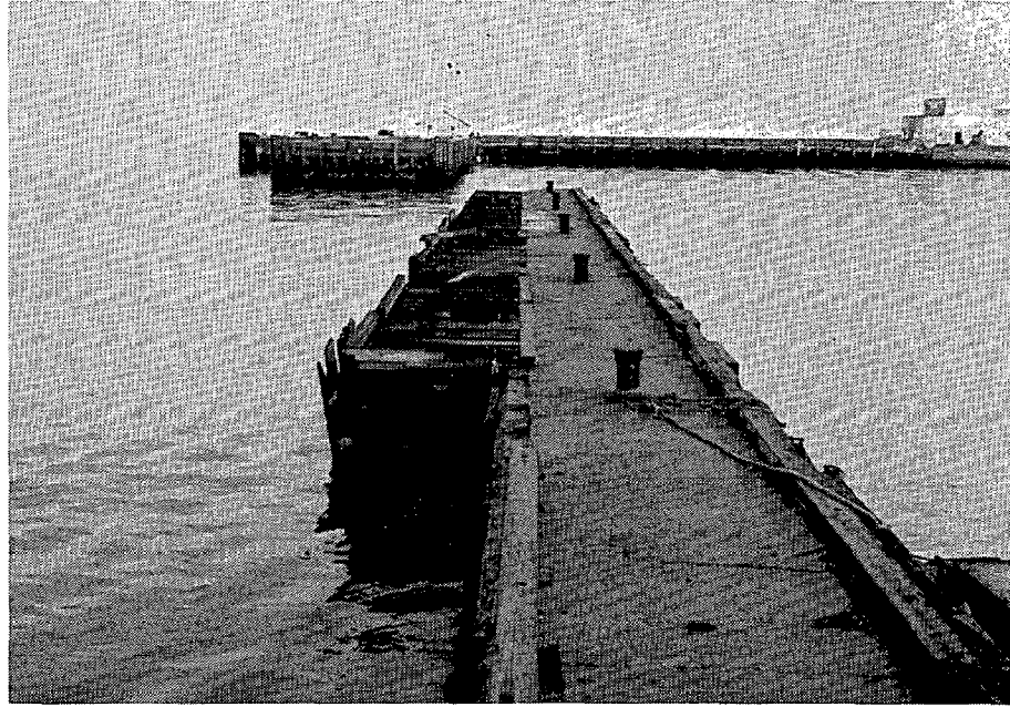
PHOTO 3 - GRANITE PIER LOCATED AT THE NORTH END OF THE SOUTH FUELING PIER. NOTE THE DETERIORATED TIMBER SECTION AND THE STEEL PIPE BOLLARDS
