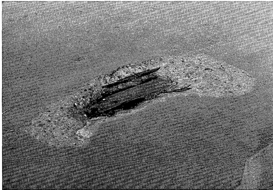
PHOTO 4 - SPALLED CONCRETE DECK AT THE FBM PIER NOTE SPLIT PIPE AT LOWER EDGE OF SPALL
