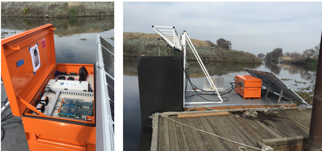
Figure 16. Electronics enclosure housing the IS1001-MC, IS1001 reader nodes, DC-DC power supply, solar charge controller, batteries, and modem positioned behind the solar panel on each raft array.
