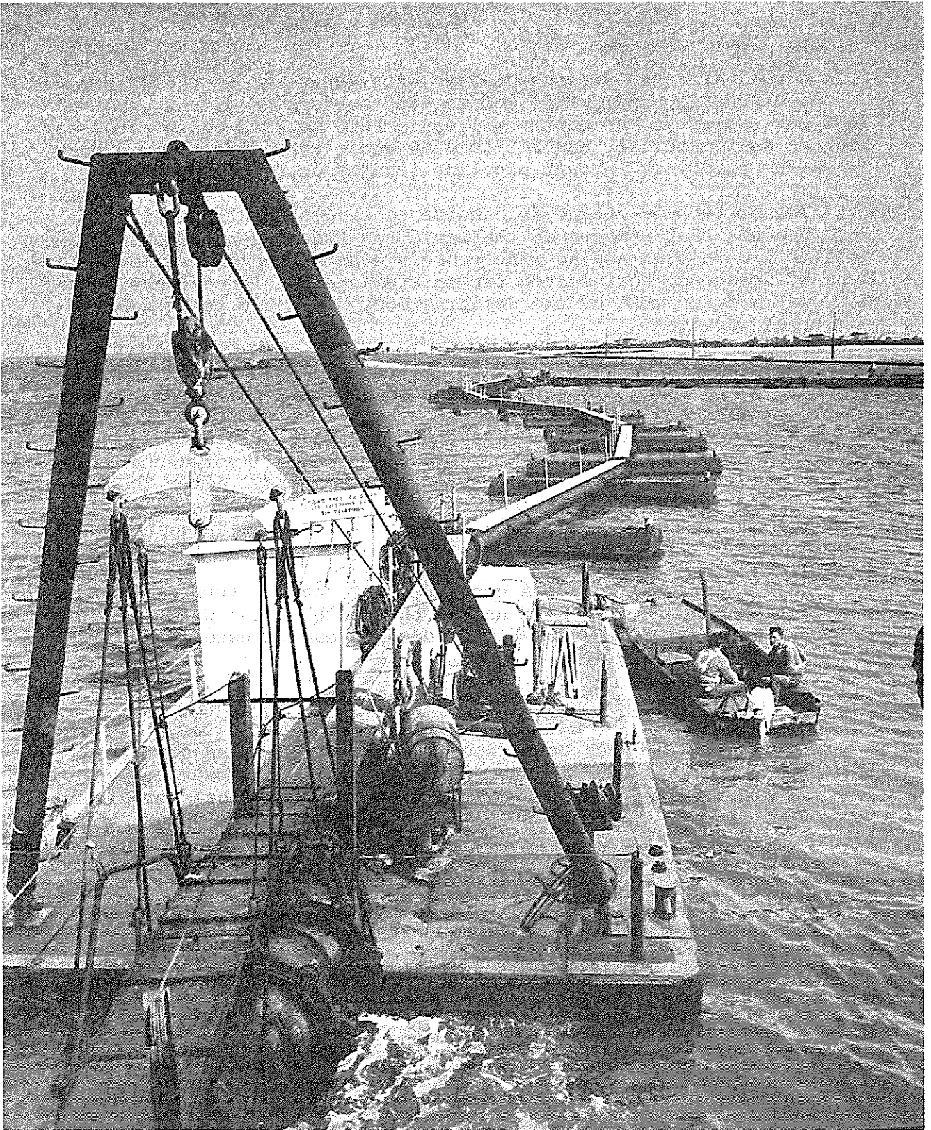
FLOATING DISCHARGE LINE (22-INCH) SHOWING BALL AND BELL CONNECTION AT THE STEM OF A DREDGE (Courtesy Williams-McWilliams Company, New Orleans, La.)
