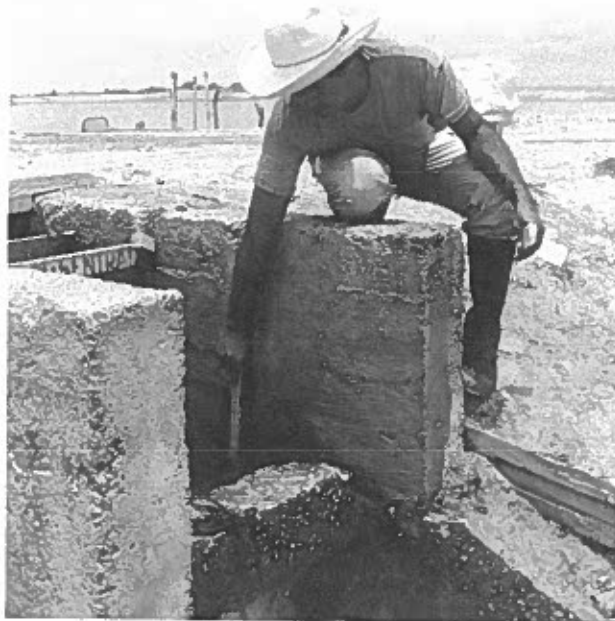
Plate 57. Personnel measuring actual water entering over entrance weir down boards. This exercise is performed in all entrance weirs at two-hour intervals.
