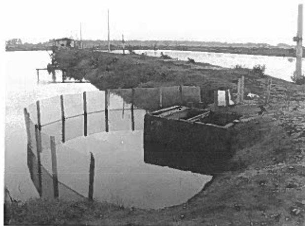
Plate 53. Semi-circular pre-filter screen installed in front of effluent gate to prevent early postlarvae from being forced against screens during strong drainage.
