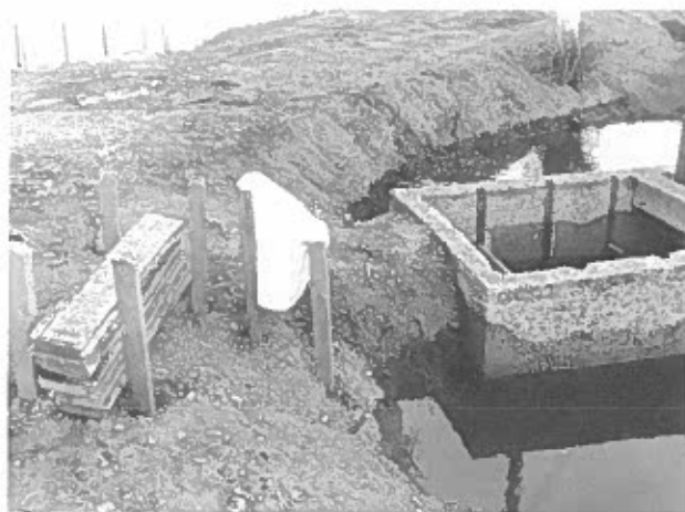
Plate 65. Empty feed bags at effluent weir gates to hold daily mortalities.
