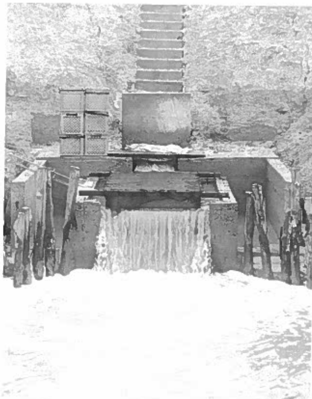
Plate 34. Down boards in place on effluent side of nursery harvest basin to maintain adequate water levels in basin and box.
