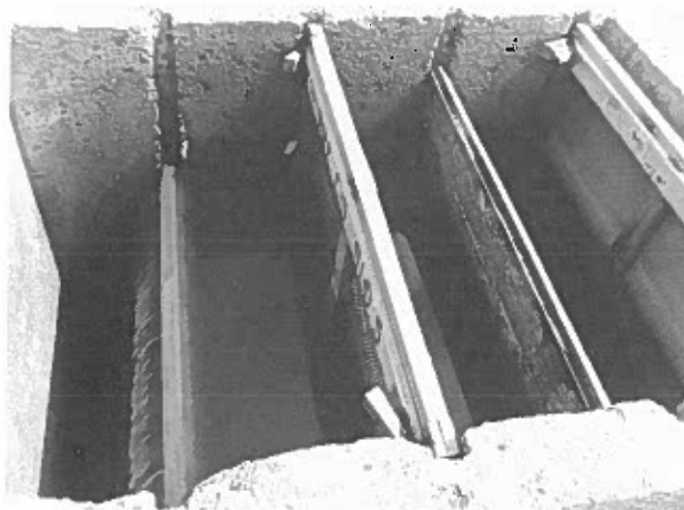
Plate 11. Screen and board configuration in effluent weir gate. Note the restriction boards in place with angle inserts to maintain pressure against board slide channel.
