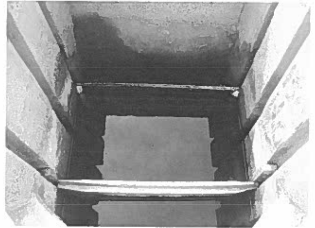
Plate 1. Boards in place in effluent weir gate sealed with the "cebo" mixture. Wedge inserts provide pressure. This set-up eliminates water seepage through board seams and edges.
