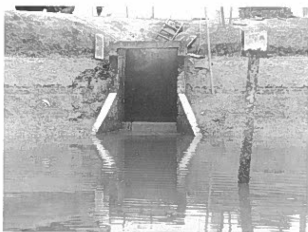
Plate 41. Flushing fresh water in reverse through the effluent weir gate to improve water quality conditions as well as increase water volume during final transfer procedures.
