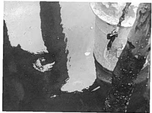
Plate 60. Whirlpool effect, at low tide, causing pump cavitation and inefficient operation.
