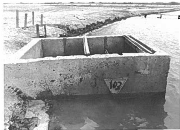
Plate 55. Operative pond water level marking triangles located on entrance weir gate walls on pond side to facilitate managing water levels in ponds.
