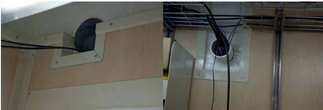
Figure 25 – Port and Aft Cabling Access Portals Inside Laboratory Space.
