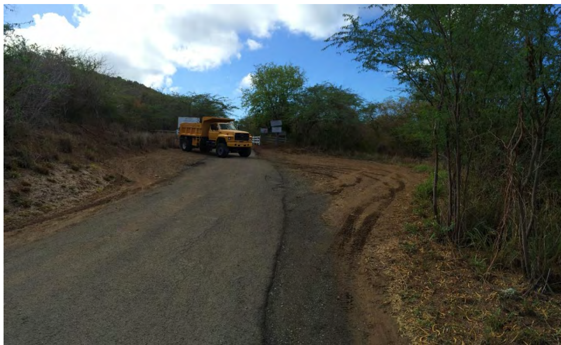
Figure 4. Picture of turnaround area of Tamarindo before stabilization.
