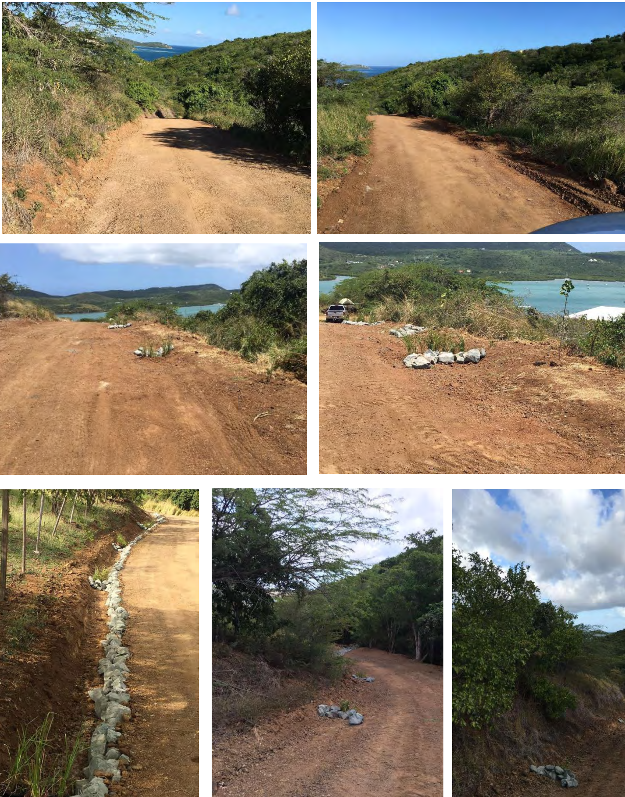
Figure 29-35. Pictures of completed dirt road stabilization with check dams in place at the Fulladosa site.
