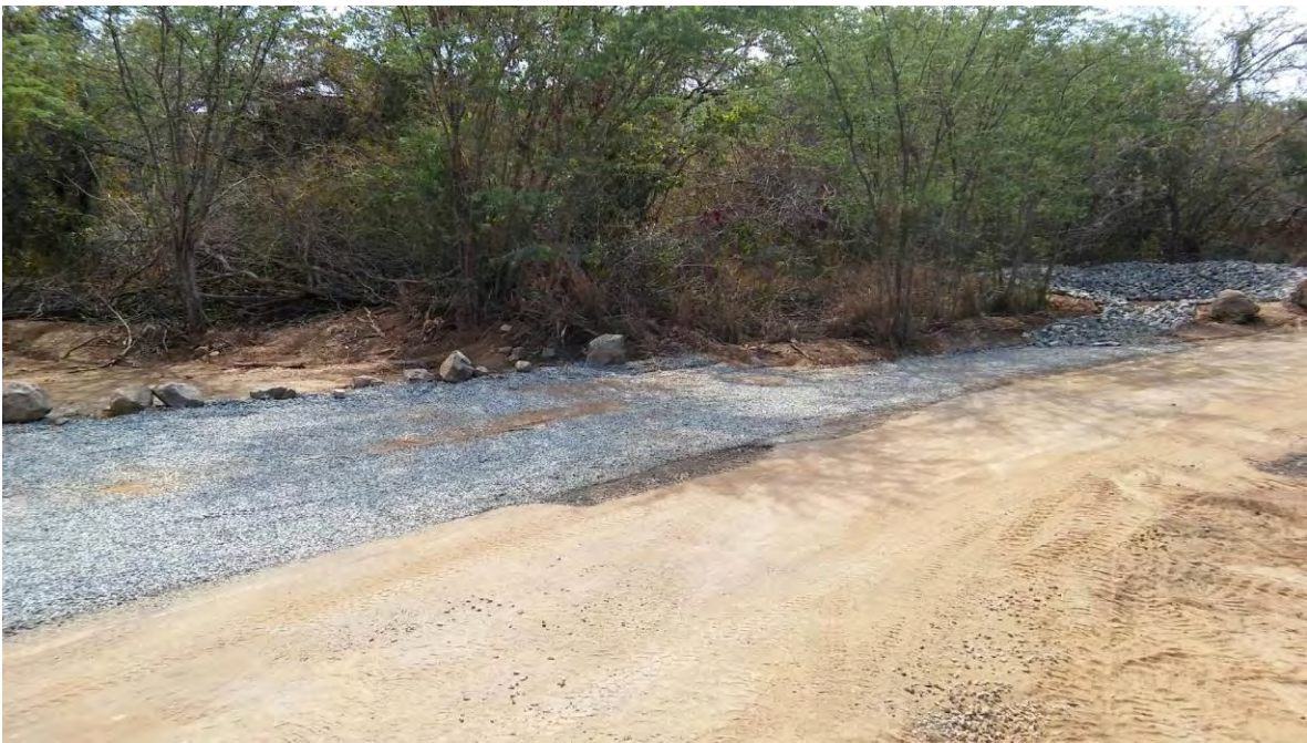
Figure 12. Turnaround site at Tamarindo after stabilization.
