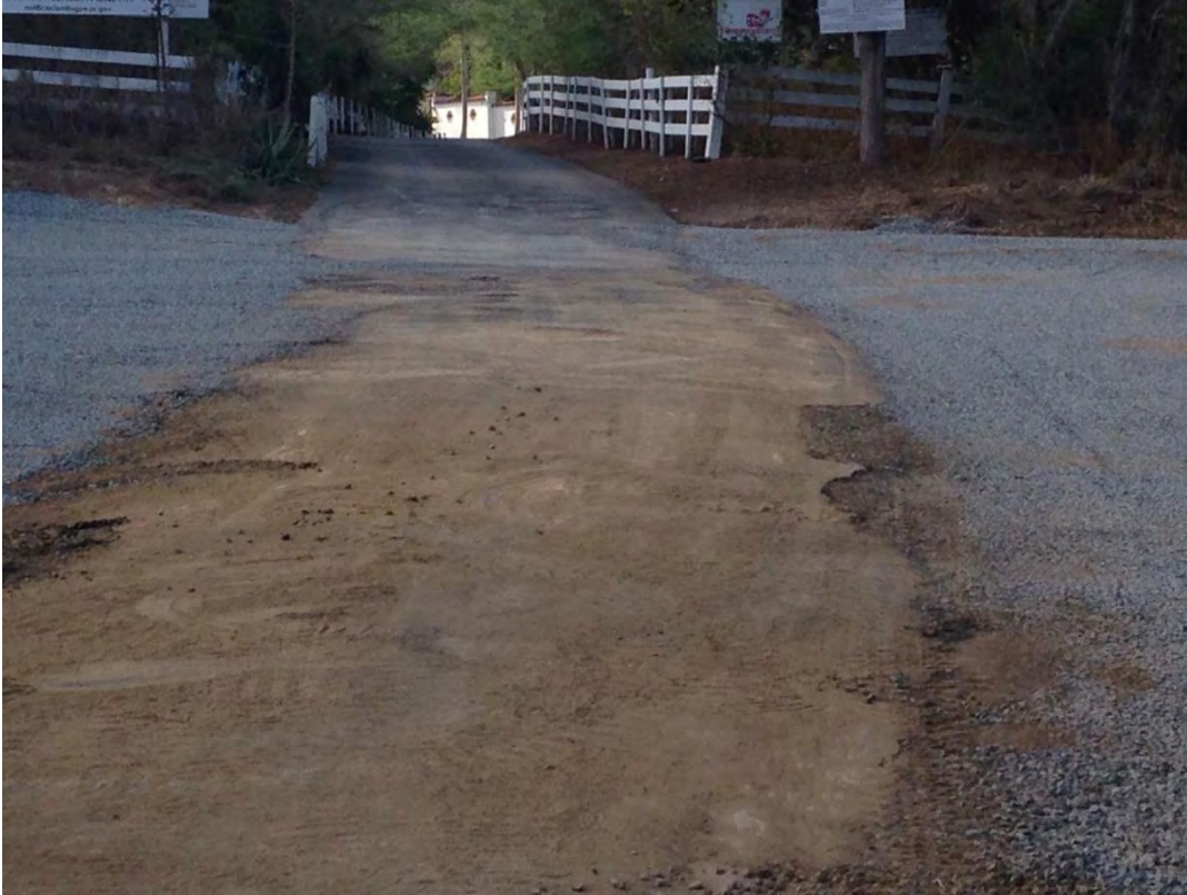
Figure 9. Turnaround site at Tamarindo after stabilization.
