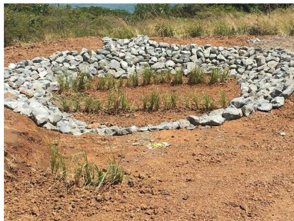
Figure 36-38. Pictures of sediment trap and rain garden construction process and completed rain garden at Fulladosa site.
