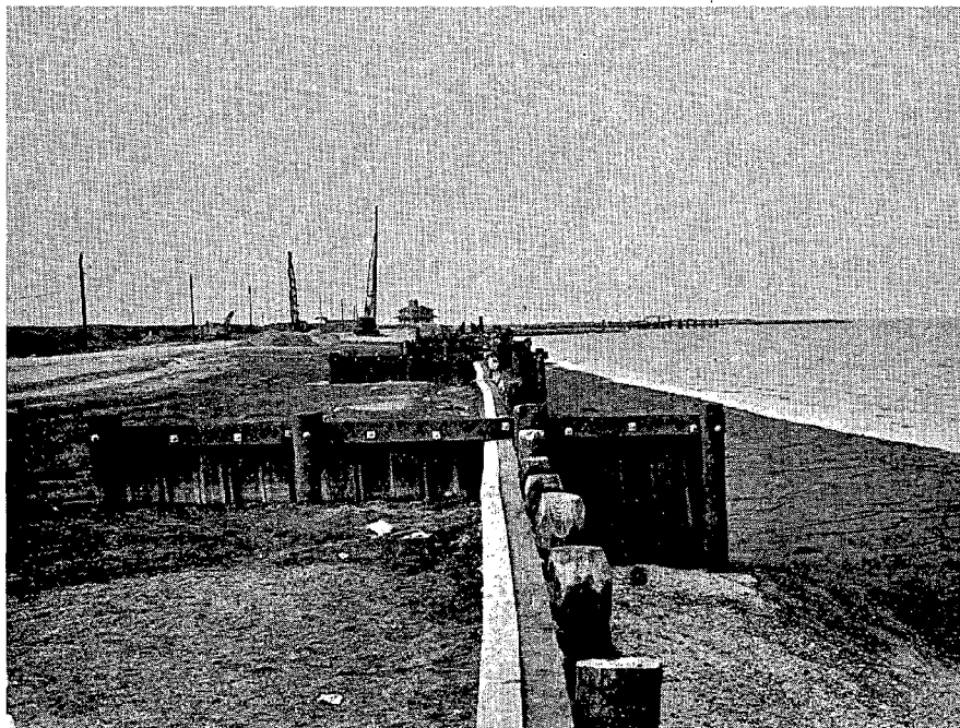
FIGURE 18. A photograph of bulkheads at Port Mahon constructed in 1975 to prevent destruction of the road by storm wave activity. (It should be noted that even portions of this barrier have recently been undermined due to wave action on the unstable mud which the bulkheads penetrated.)
