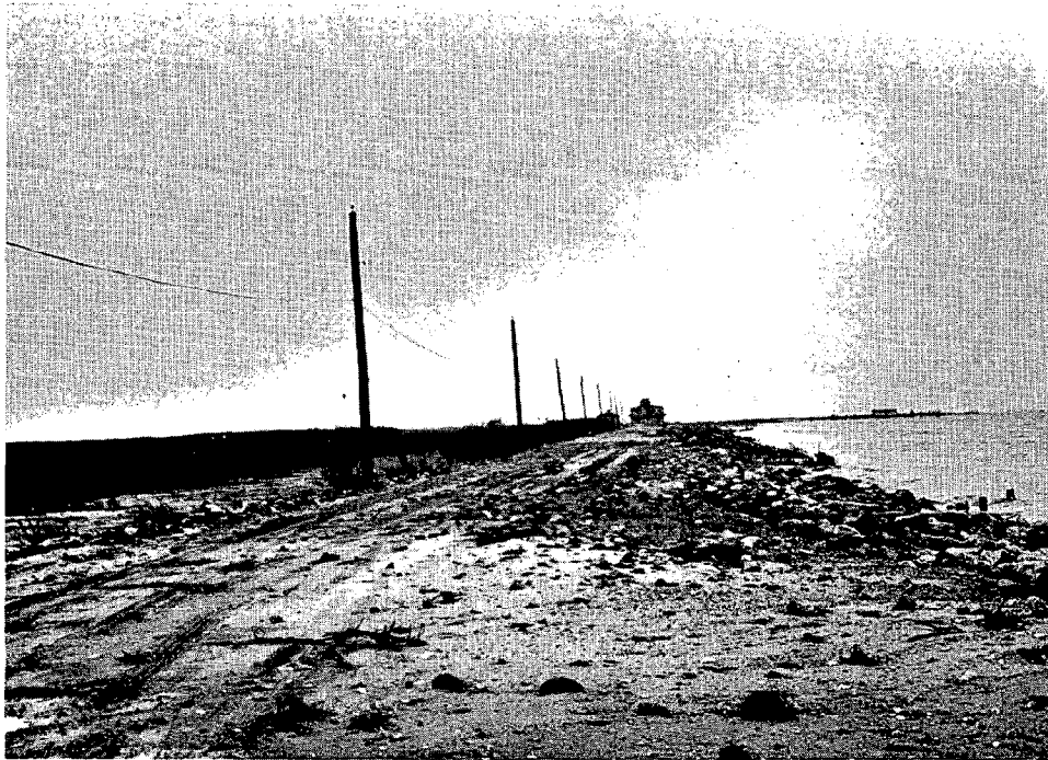
FIGURE 17. 1973 photograph of the shoreline at Port Mahon showing the road washed out and covered by sand and debris.
