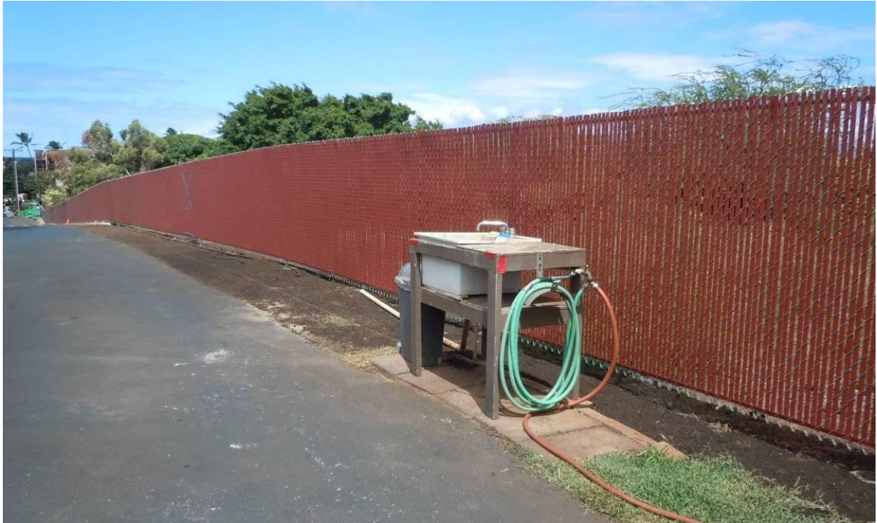
This utility sink next to the laundry building at Hale Royale discharges on exposed soil and then down the steep driveway to a catch basin at the intersection with Lower Honoapiilani Hwy.
