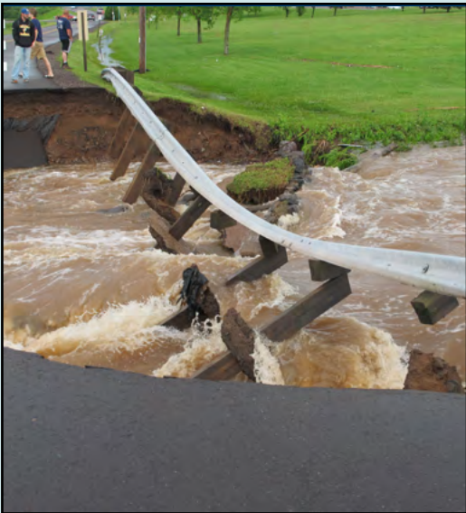
Flooding at Flaxon Creek in 2012. Credit LSNERR.
