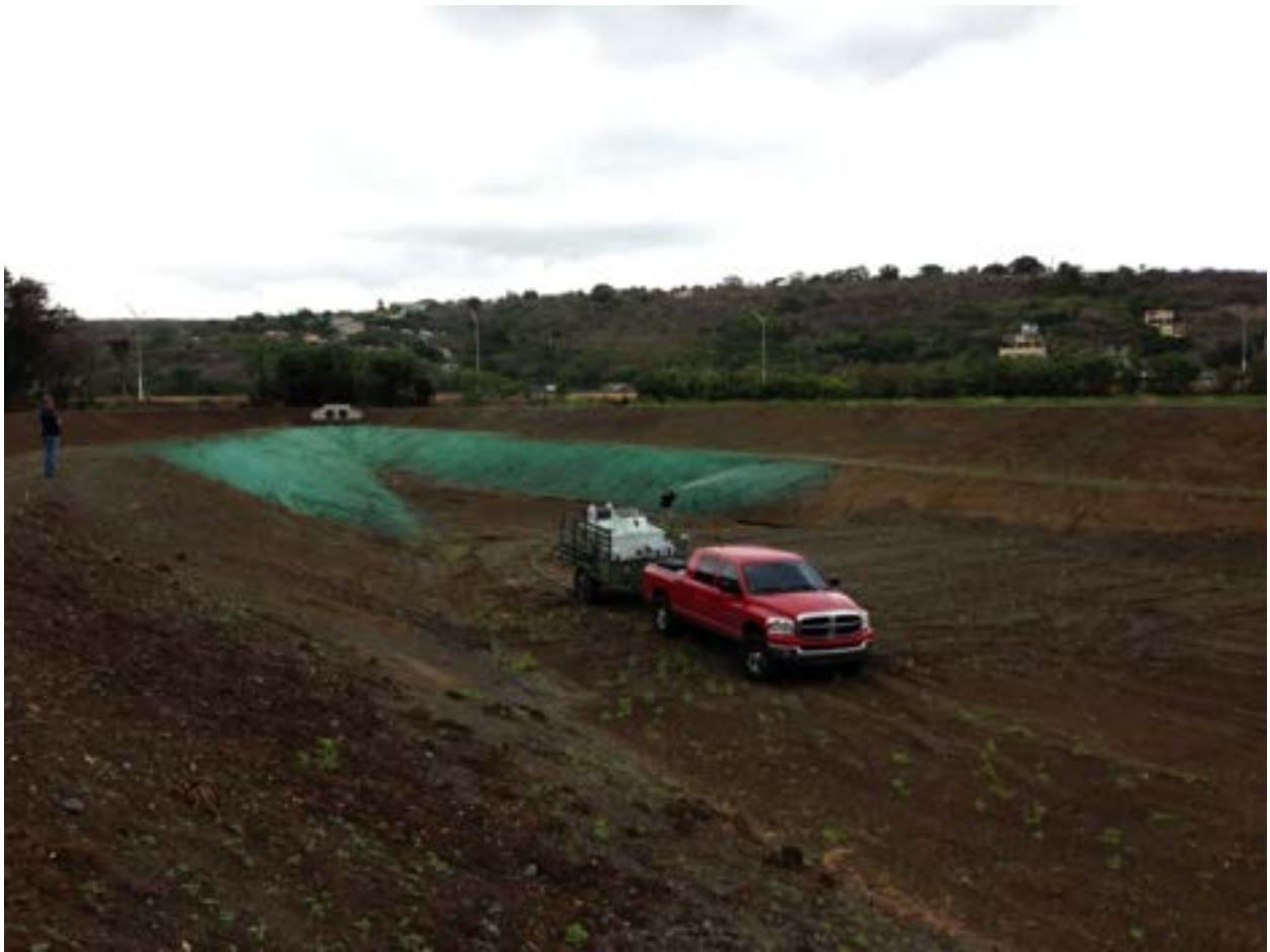
Figure 3. Hydromulch application in the sediment basin working with the Southwest Soil Conservation District and NRCS
