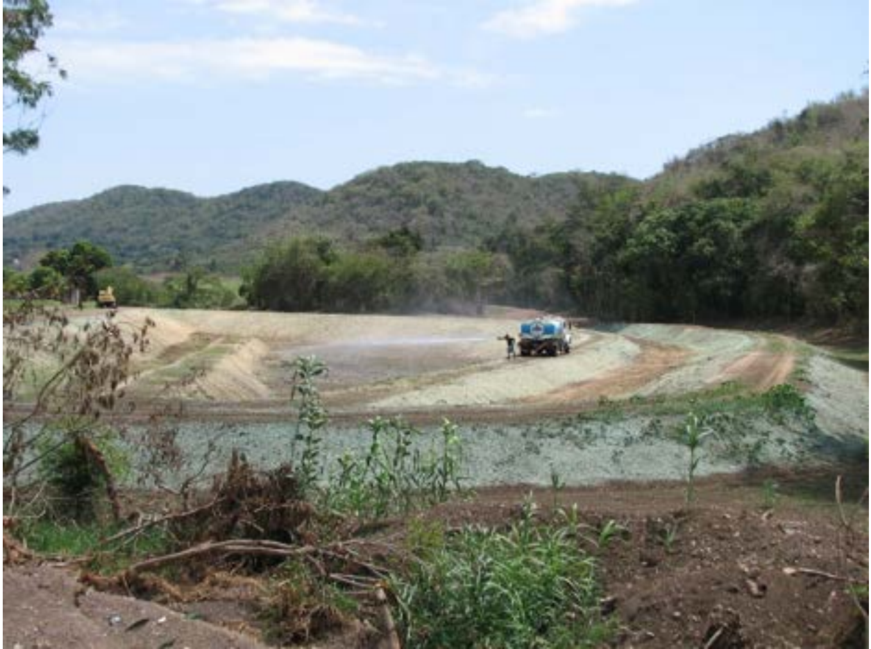
Figure 4. Watering the sediment pond project site using assistance from Department of Natural and Environmental Resources
